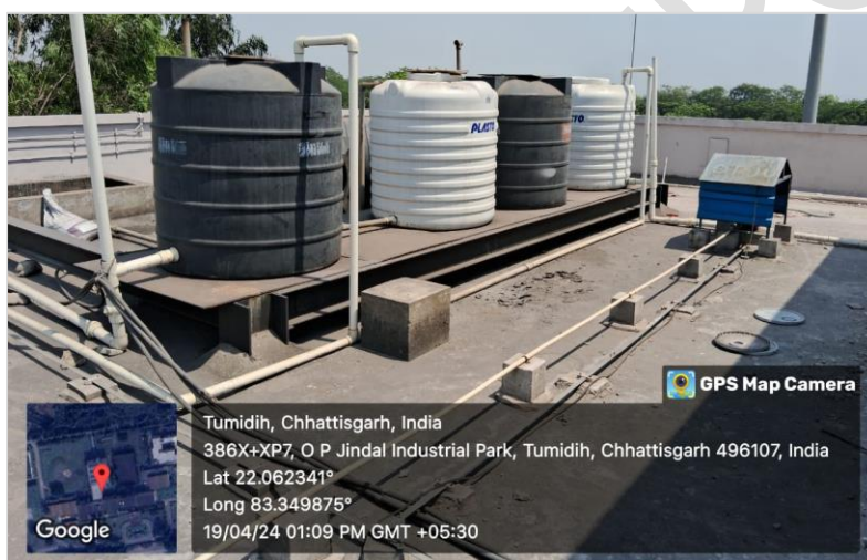
Plate 1: Water tanks on the rooftop areas
